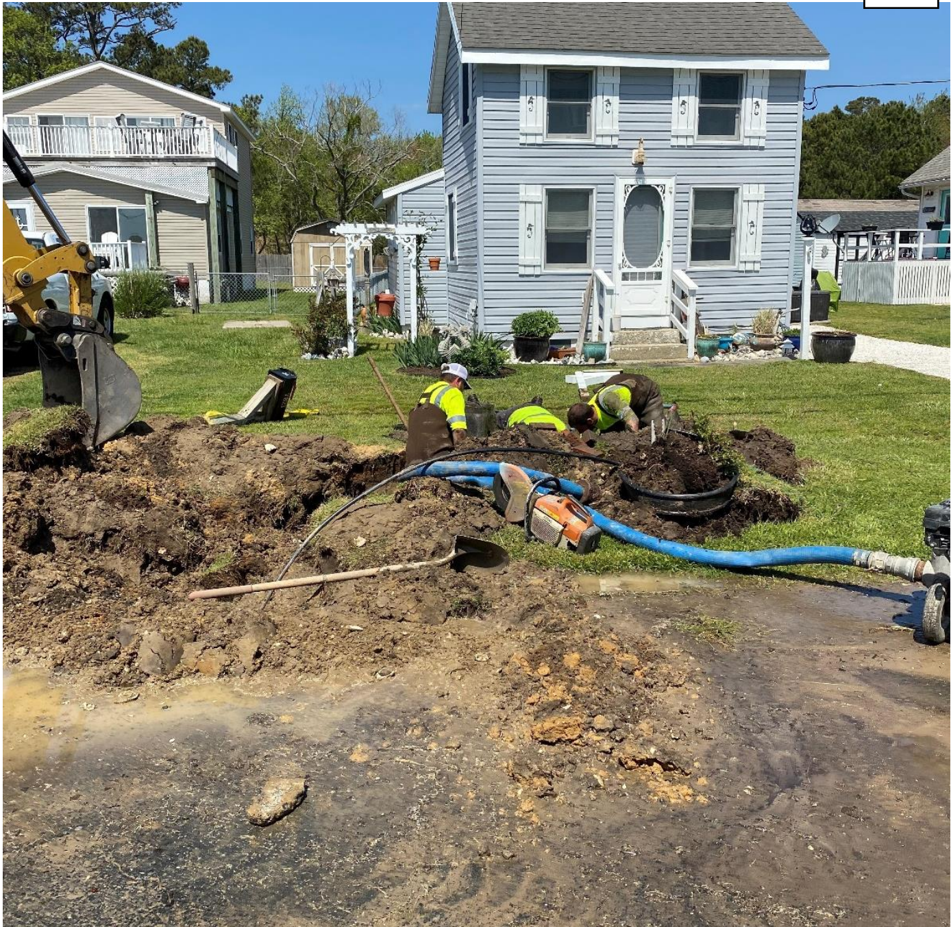
Water Main Leak East Side
